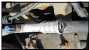
Damaged A/C Line
