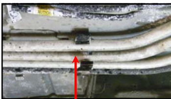
Rusted A/C Line
